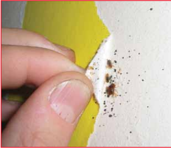
• Inspect behind loose wall paper
