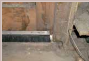
INCORRECT USE OF BRISTLESTRIPS
